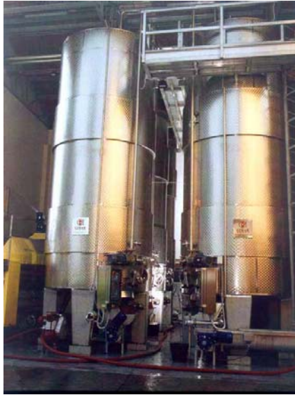
Cuve Gimar Selector System (sourceGimar)
